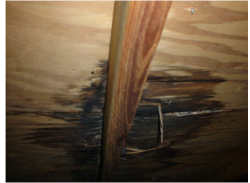
Photo # 5 ROOF LEAK AS OBSERVED FROM ATTIC
